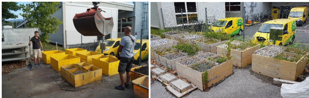
Figure 2: Installation of the test boxes in Villach at the campus of the Carinthia University of Applied Sciences. (Wiegele)
